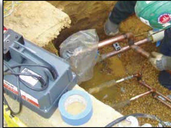
This outside installation used Lokring couplings to connect existing medical gas lines to new lines for hospital expansion. This installation included 3/4 in. size for nitrogen and nitrous oxide. The oxygen line was 1 1/2 in. size on Type L copper. The total installation time for the three fittings was 20 minutes.
